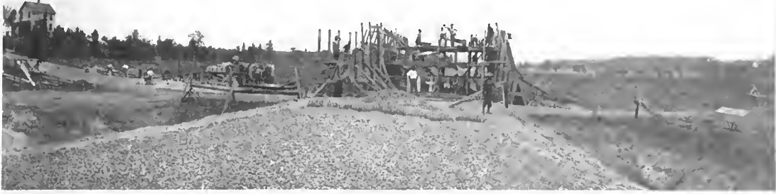
Showing the Wooden Molds, Mixing Machines for Cement and Stone, and Wire Netting Which Goes Between.
